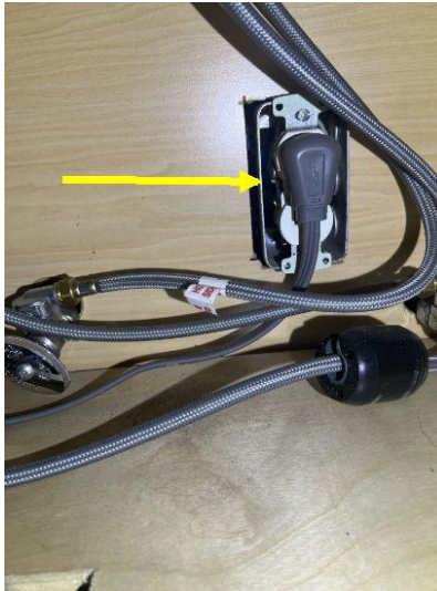
Missing cover plate under sink
