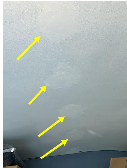
Patching in bedroom ceiling
