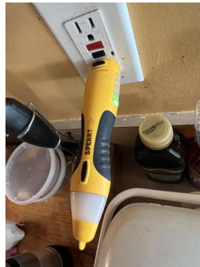
Kitchen - GFCI DID NOT RESET
