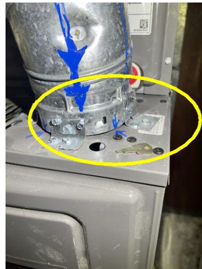
Air is leaking at the duct connections. These should be checked and sealed for energy conservation.
