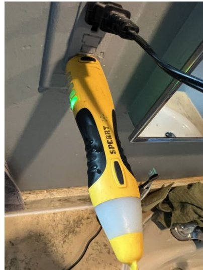
Bathroom - GFCI DID NOT RESET
