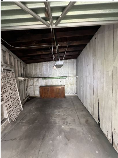
Unit 3 - Staining along wall
