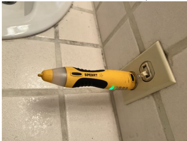
Bathroom - NO GFCI
