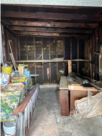
Some garages have windows that are missing the glass. They are boarded up.
