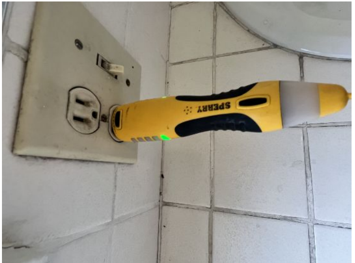
Bathroom - NO GFCI
