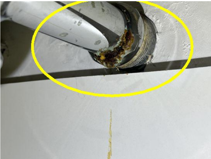
The drain line is corroded and leaking.
