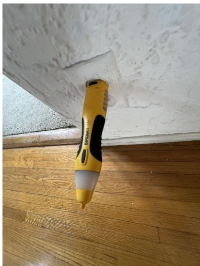
Unit 4: There are outlets that are dead and not working - Unit 4
