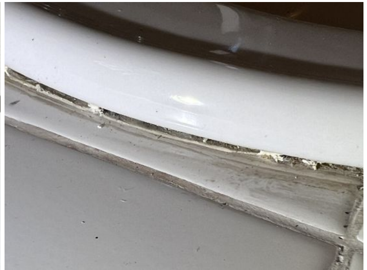
Sink seal is deteriorated.
