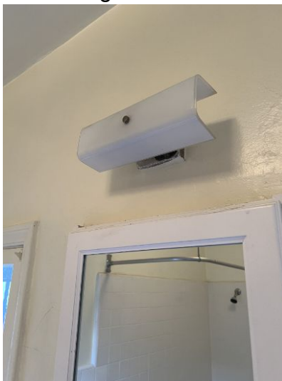
Fixture does not operate
