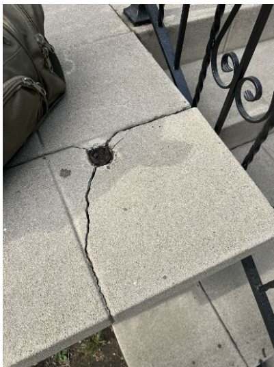
Cracked cement tile near the front stairs.
