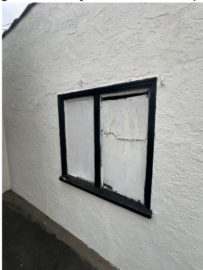
Some garages have windows that are missing the glass. They are boarded up.
