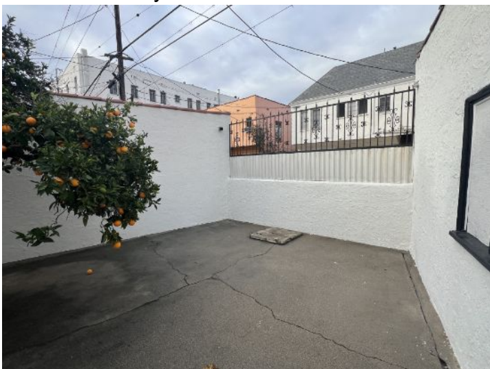
This area drain is full and overflowing.
