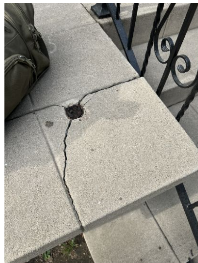
Cracked cement tile near the front stairs.
