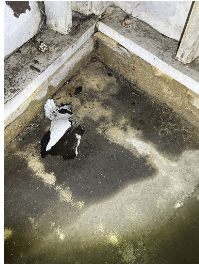
Moisture on the floor.
