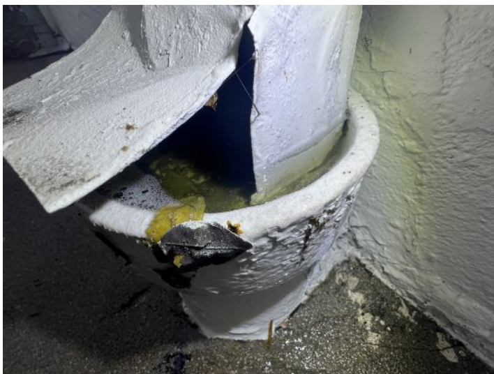
This area drain is full and overflowing.
