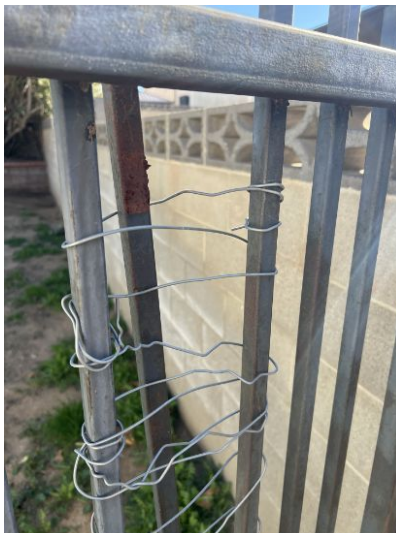
Damaged gate - right side
