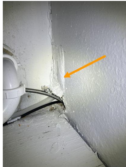
There are some areas where there have been temporary "fixes" for things. It appears that non-standard repair practices were used when these fixes were made. - Under kitchen sink.
