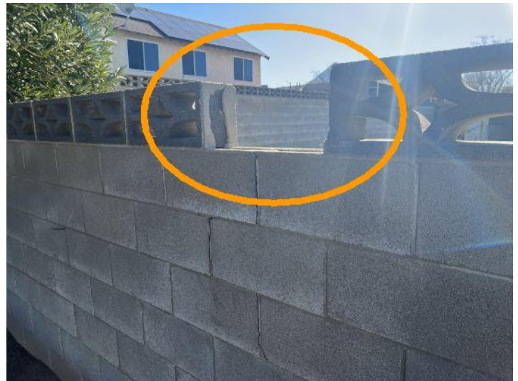
Damaged block wall
