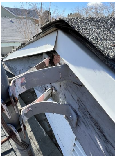
Roof antenna is pulling away from bolting / fascia.
