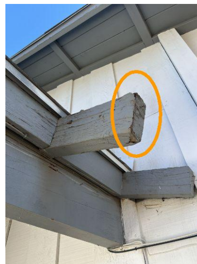
The rafter tails are deteriorated in areas.
