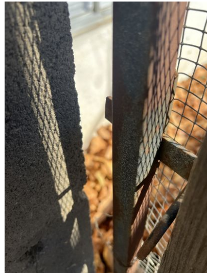
Right side gate - missing locking mechanism
