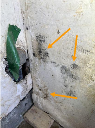
There are areas of possible mold and mildew observed on the water heater stand. This can be cleaned locally or replaced.
