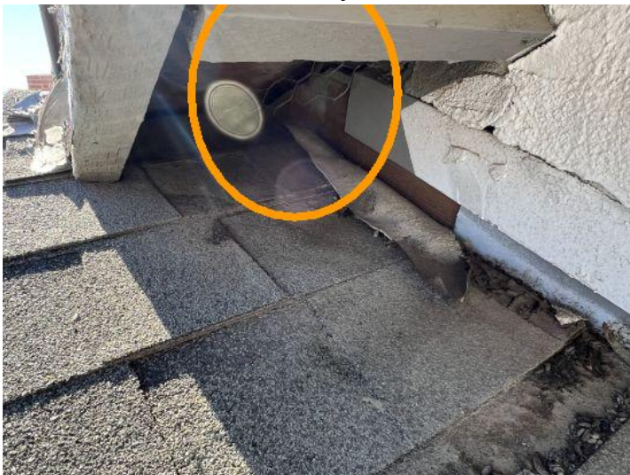
Area is open to the attic.
