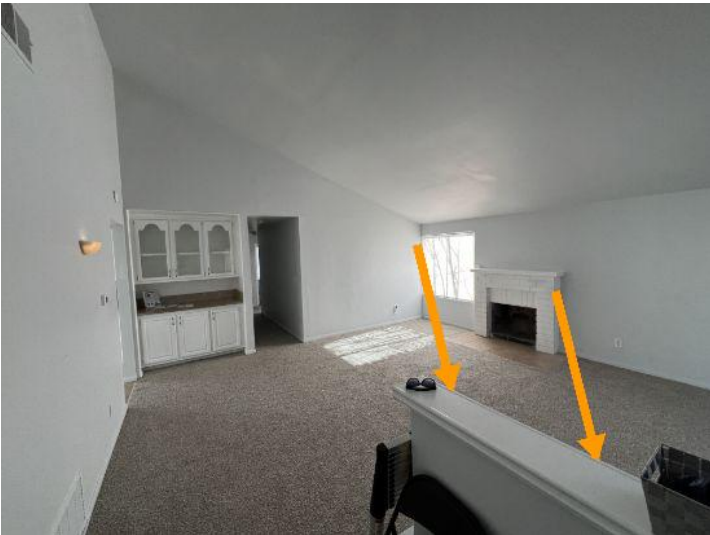
The decorative pony-wall at the entry is not secured properly and is loose.
