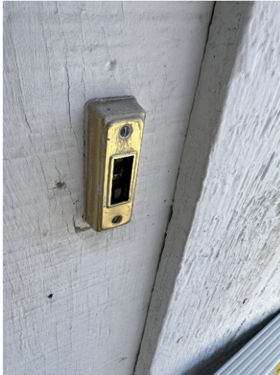
The doorbell ringer is missing some parts.
