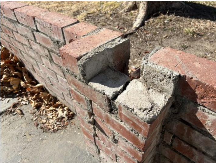
There are garden brick walls that are leaning, missing bricks and/or have step cracking in them.
