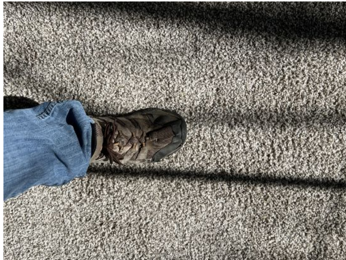
Crack felt in floor - living room
