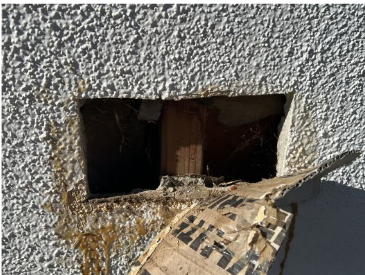
Hole in exterior - covered with cardboard.
