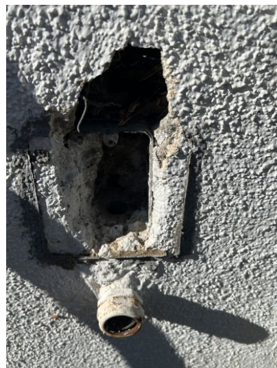
Hole in exterior
