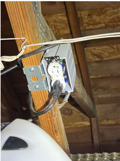
No coverplate - in garage.
