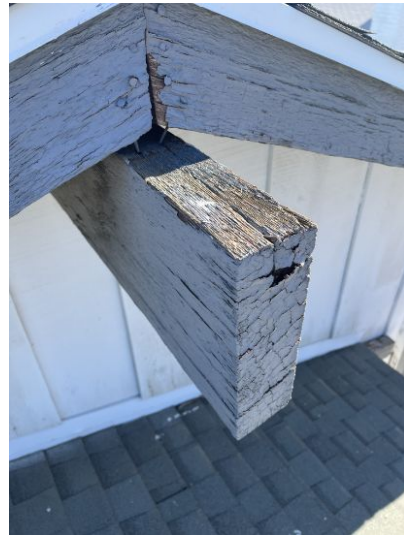
The rafter tails are deteriorated in areas.
