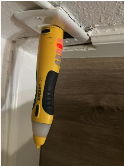
Under stairs - NOT GROUNDED PROPERLY
