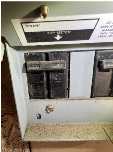
Because they are not marked, it is unclear which one belongs to Unit A
