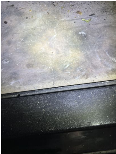
Gas line is capped
