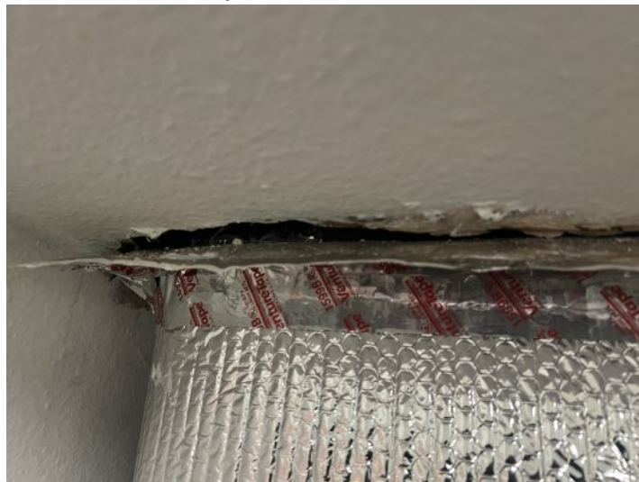
Not sealed properly
