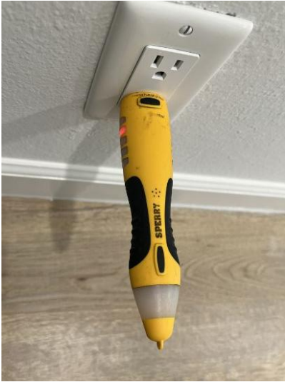
Bedroom 2 - NOT GROUNDED PROPERLY
