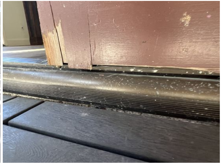
There are exterior doors that have some deterioration.
