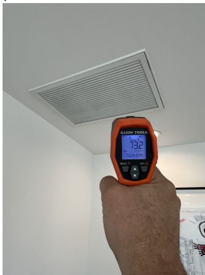
Upstairs - 73 deg F - return air
